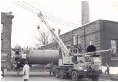
Installation of Boiler in Chemical [Engineering] and Centre for Energy Studies Building, c1972-1973
