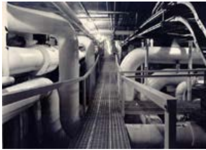
Central Services Building - Pipes, n.d.
