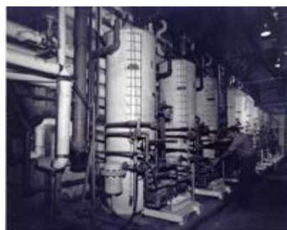
Central Services Building - Boiler Room, n.d.
