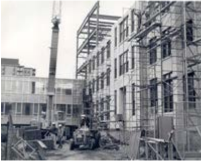
Macdonald (D) Building under construction during the building of the Nova Scotia Technical College's new administration complex, c1960-61
