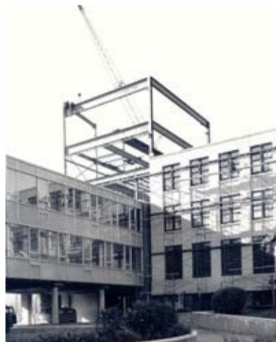
Macdonald (D) Building under construction during the building of the Nova Scotia Technical College's new administration complex, c1960-1961
