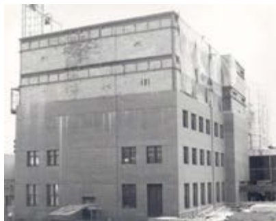
Macdonald (D) Building under construction during the building of the Nova Scotia Technical College's new administration complex, c1960-61
