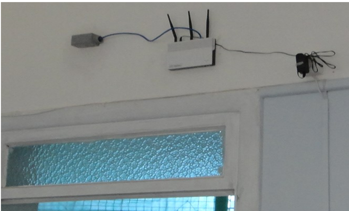
Figure 5: Wi-Fi Installed High in Hospital
