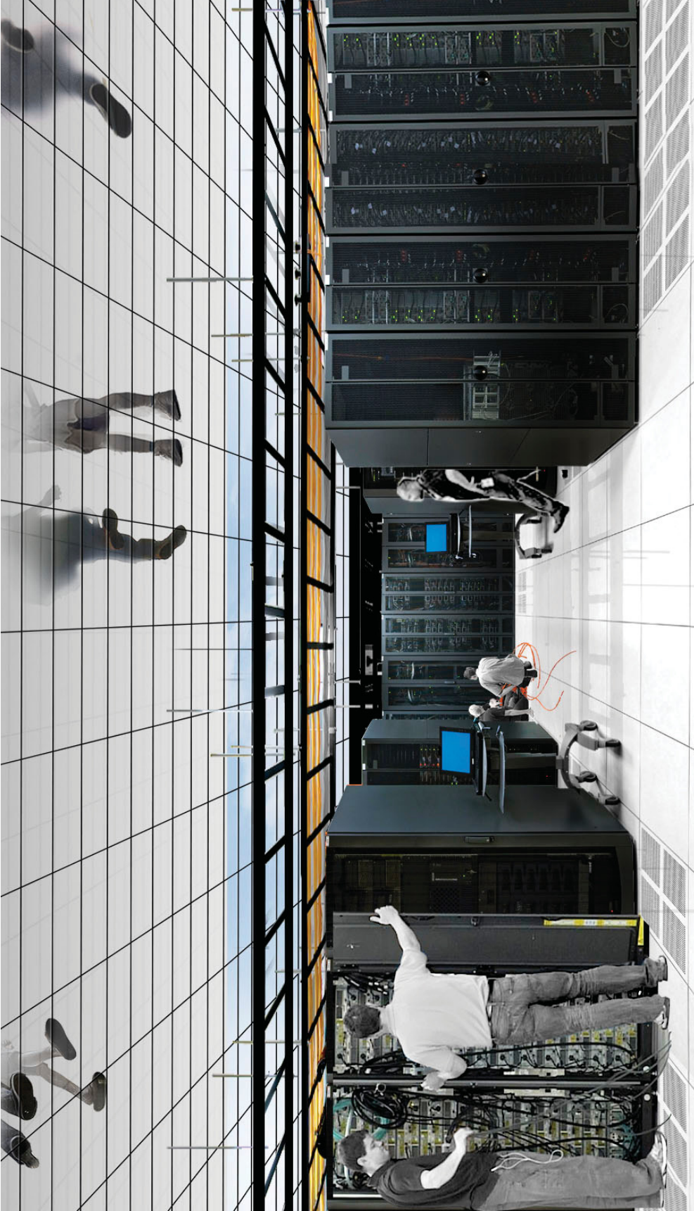
Data centre technicians maintain the machines holding private data while the public operates on the public square above
