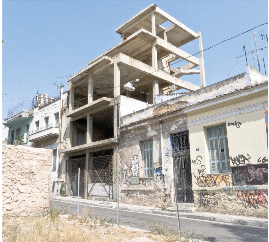
Figure 12: An unfinished polykatikia in Metaxourgio, revealing the free plan of this typology, 2011
