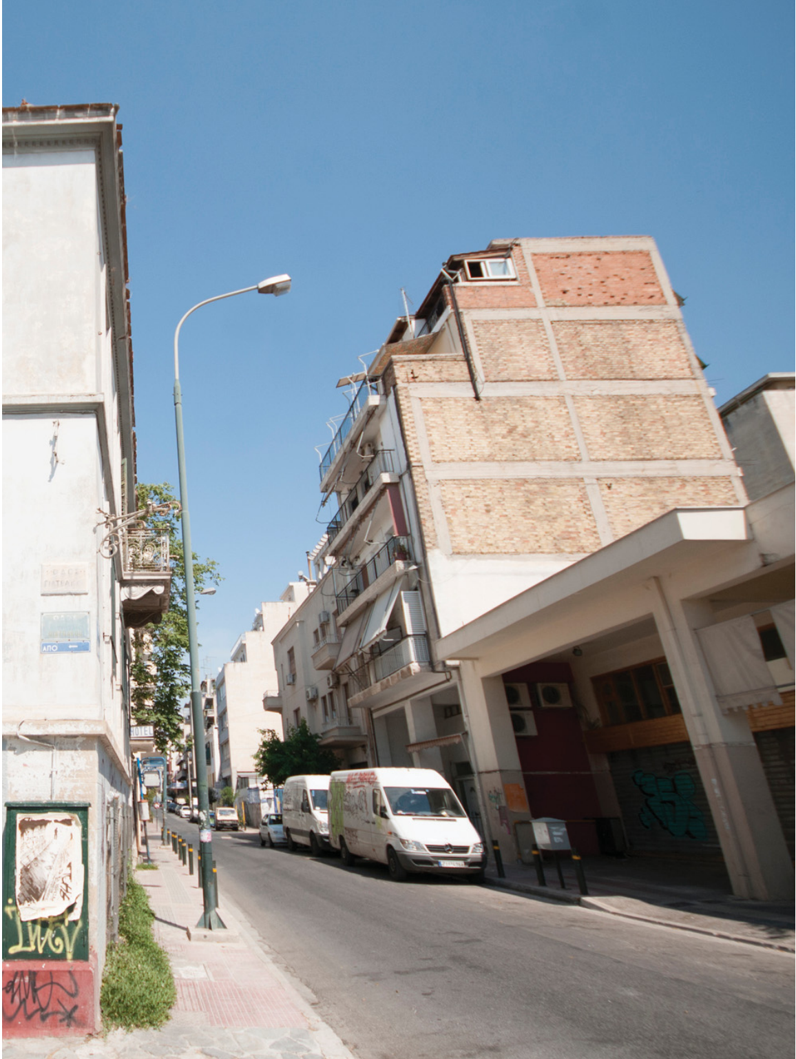
Figure 43: An unfinished parti wall reveals the wall construction as infill between the concrete structural frame, 2013
