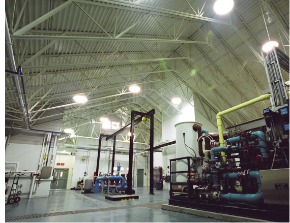
Wasagaming water treatment plant interior, 2004; from Bird Construction
