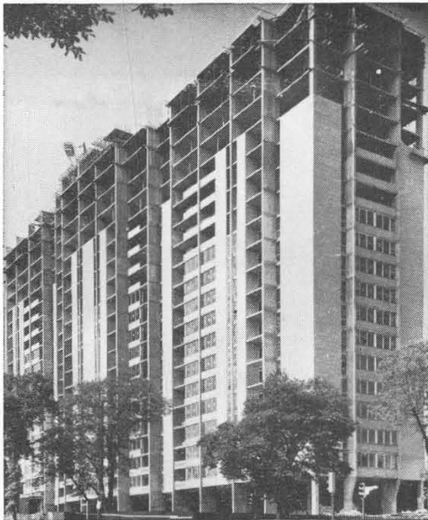
Park Victoria Apartments, Halifax, N.S. Architects: Elmar Tampold and J. M. Wells. Consulting Structural Engineers: Blauer, Horvath, Desjardins Associates. General Contractor: Croy Construction Ltd. Ready-mixed concrete supplied by: Hubley's Sand & Gravel Co. Ltd.
