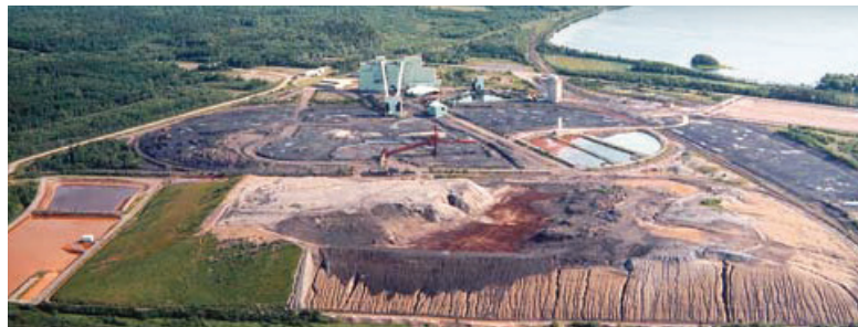
Victoria Junction - facility dismantled, but before remediation. Source: Public Works and Government Services Canada.
