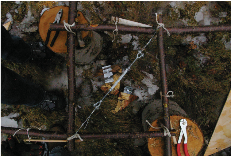
Steel cable with a turnbuckle used to tighten the connection
