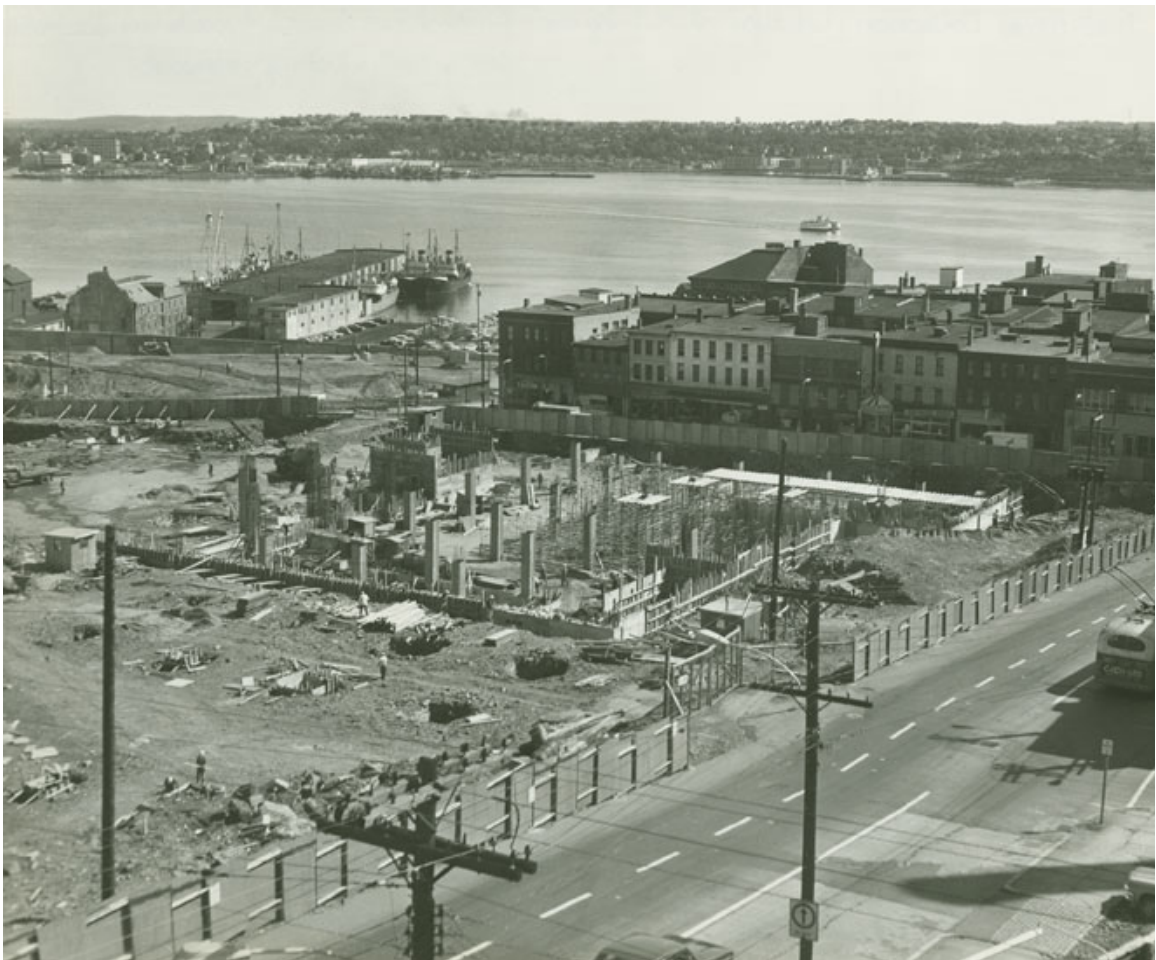
16 acres were demolished for the urban renewal scheme. Pictured here is the corner of Duke and Barrington Street where the mixed use, commercial, Scotia Square was to be built. (NSA 1967)
