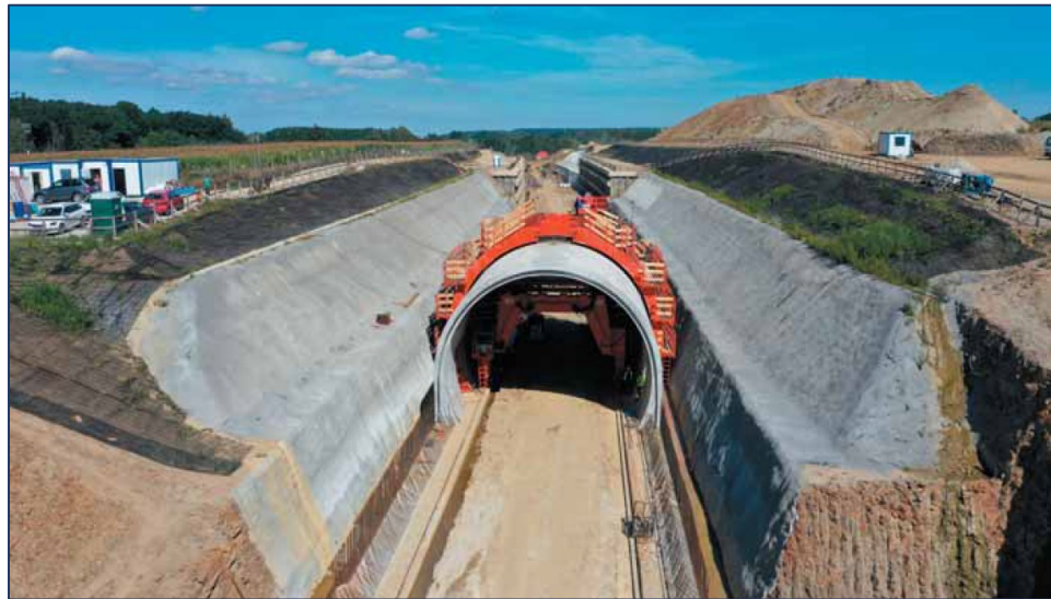
Figure 1-1: Excavation of trench and installation of concrete lining for a cut and cover tunnel construction (Zvěrotice Tunnel – Overall View)
