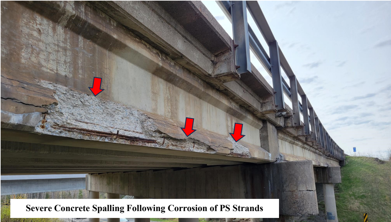
Figure 2- Severe corrosion-induced spalling of a prestressed concrete bridge girder, NS
