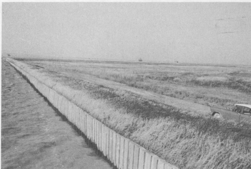
Figure 10 – Aulac Marsh – Another common method of protecting exposed dyke from wave erosion during high tides. (Photo 24 - 020) - 1961
