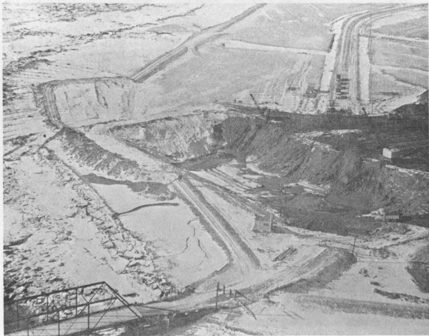
Figure 7.-- Nappan River Dam, Cumberland Co., N.S. Excavation in progress for a two barrel 10ft. X 12½ft. concrete sluice. A rock fill causeway will replace the bridge at lower left.
