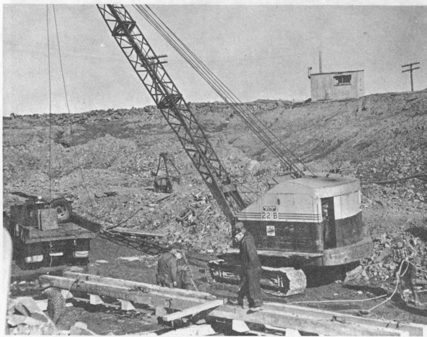
Figure 8.-- Nappan River Dam. Preparing leads for driving pile, necessary to support the reinforced concrete sluice.
