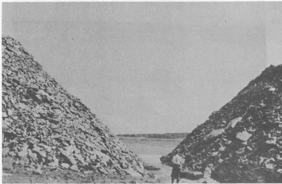
Rock fill, just prior to closure at low tide, during construction of the large aboiteau at Noel Shore. This structure eliminated the need for rebuilding other aboiteaux and adjacent dyke and also reclaimed an area of marsh which would not otherwise be protected.
