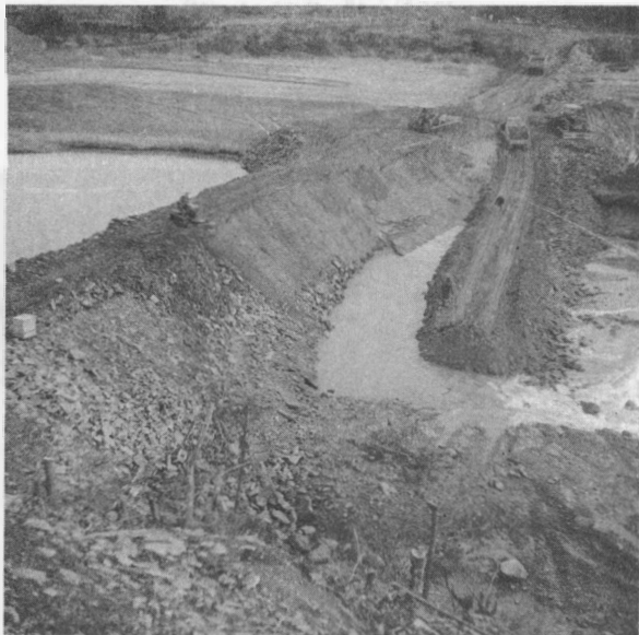
Placing of the fill in the second aboiteau protecting New Horton Marsh. Rock fill is being advanced on the downstream portion of the fill. A core of fine material was placed to reduce and almost eliminate the flow through the fill as shown above. The sluice shown in the previous photo is located below the cut bank in the very immediate foreground.
