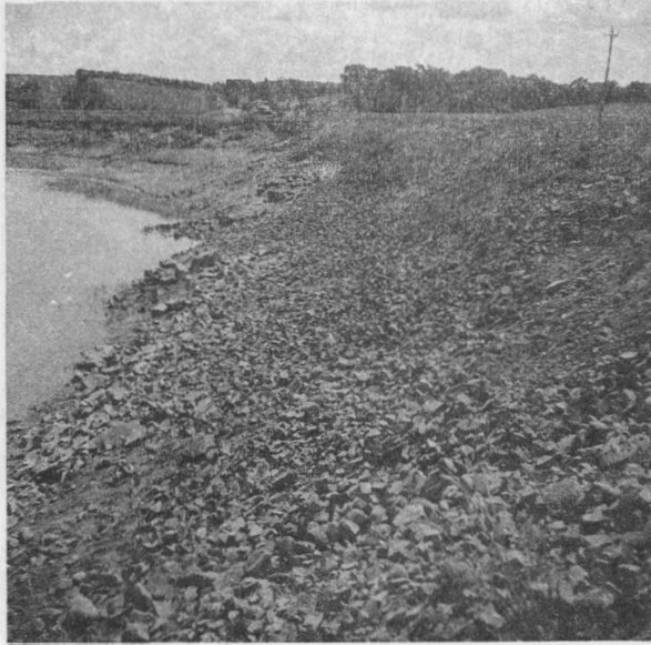
Mantua-Poplar Grove Marsh, Hants Co., N.S. — Rock facing placed to prevent undercutting of the road grade which also serves as a section of dyke to protect this marsh.
