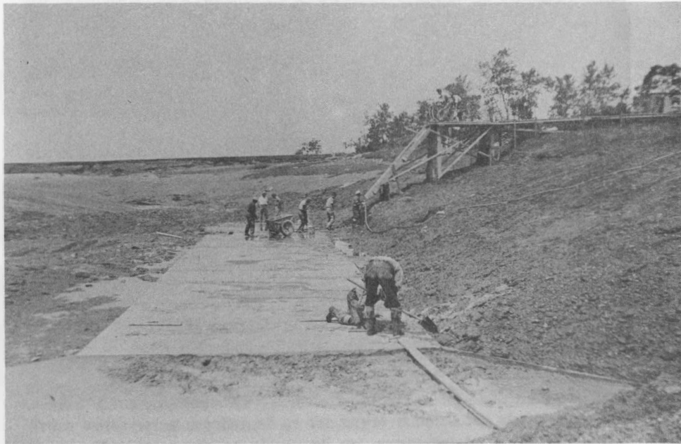
Noel Shore Marsh, Hants Co., N.S.—Advantage was taken of a rock ledge by using it as a foundation for the aboiteau sluice. Normally sluices are set on marsh earth foundations, rock ledges not being common. A cement bed was laid and the timber sluice anchored to it and the rock formation below.
