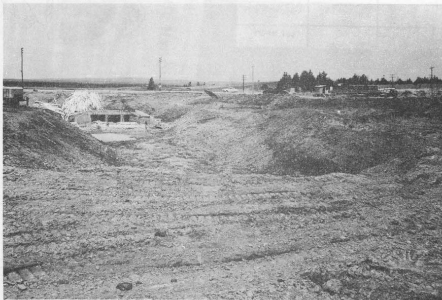
The partially completed Isgonish bridge-aboiteau in the spring of 1955. Highway traffic is running over the new sluiceway and the Bailey Bridge is still being used to cross the old river channel. This old channel will be blocked and flow diverted through the new structure shown here. This new structure will be equipped with gates to allow fresh-water drainage during low tides and to prevent salt water from entering the valley during high tides. (Photo N. S. 15/100).
