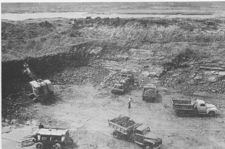
Machines engaged in the excavation of the Shepody River Project spillway during the summer of 1954. This spillway or sluiceway is located in the south bank of the River behind the old Harvey Bank Wharf. Cofferdams are being maintained at either end of this sluiceway until the piers and control apparatus are completely installed in the excavation (Photo N. B. 51/214).
