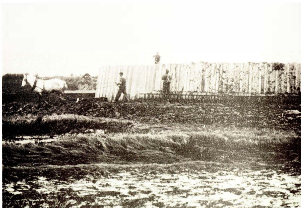
Fig. 10 - Project N. S. 8, Grand Pre Marsh, N. S. A section of vertical plank facing being installed. This is necessary in those locations where the dyke is exposed to severe wave action. Normal tides flood the marsh in the foreground almost daily, but it is the higher tides which necessitate the plank facing.
