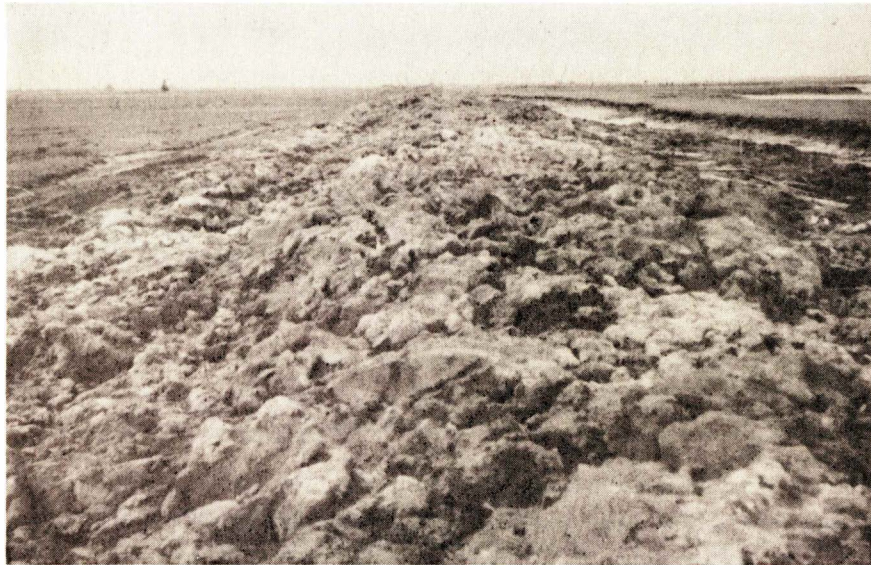
Fig. 1 - Project N. B. 5 - Westcock Marsh, N. B. A section of dyke under construction. A dragline cast the fill from the borrow pit at the right. Final grading remains to be completed.
