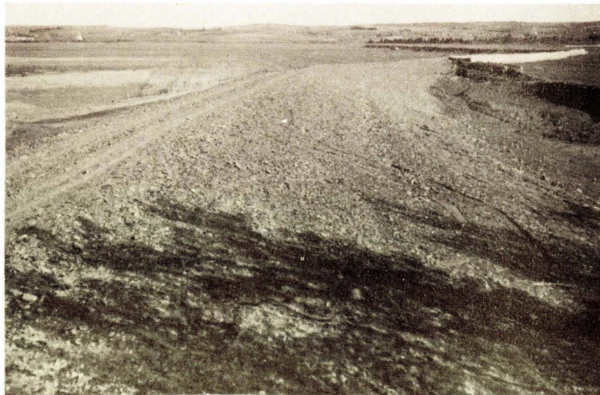
Fig. 8 - Project N. S. 8, Grand Pre, N. S. This is a view of an aboiteau on which pit run gravel has been placed to provide protection against tide water action. This aboiteau was installed to replace one which was near collapse.
