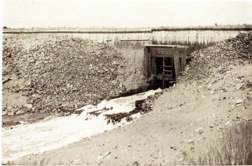
Fig. 13 - Project N. S. 41, Habitant Marsh, N. S. This aboiteau was completed in 1945. However, the heavy discharge of fresh water necessitated the extension of the aboiteau discharge spillway to prevent undermining of the entire structure.
