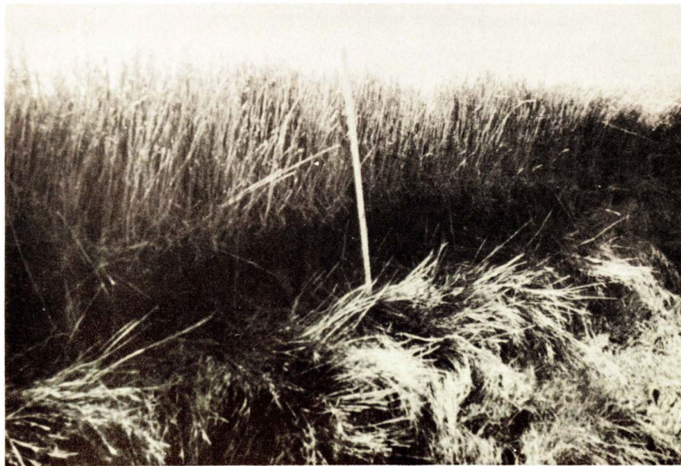
Fig. 4 - Project N. S. 5, Dugau Marsh, N. S. This view shows a section of dyke where the tide water has caused erosion near the top of the dyke and overtopping or breaking of the dyke is very likely to occur. It is a typical condition of many of the protective dykes.
