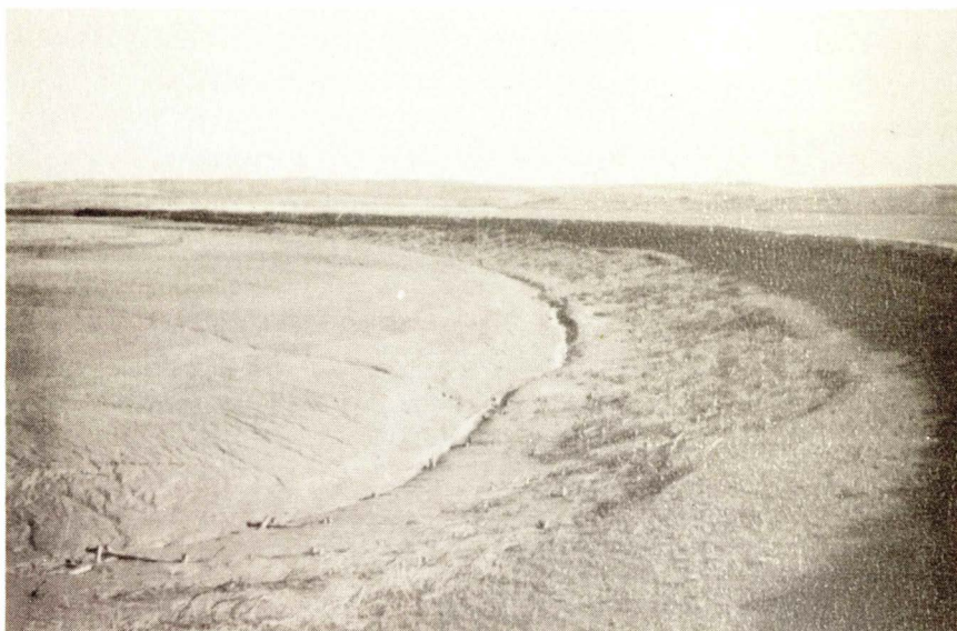
Fig. 9 - Project N. S. 8, Grand Pre Marsh, N. S. The tide water flowing up and down this gully tended to undercut the dyke. To provide protection which would not necessitate the setting back of the dyke, brush matting was placed as shown. The effect has been to move the gully channel to the left as well as to encourage silt deposits and bank build up.
