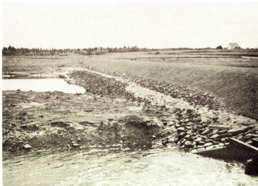
Fig. 18 - Project P. E. I. 1, Johnston River, P. E. I. This fill, forming a part of the aboiteau, is made of rock and earth without the benefit of a brush mat foundation or brush in the fill itself. It is believed to be the first of its type erected. Rock rip-rap has been placed on the down stream side to prevent damage from tide water.
