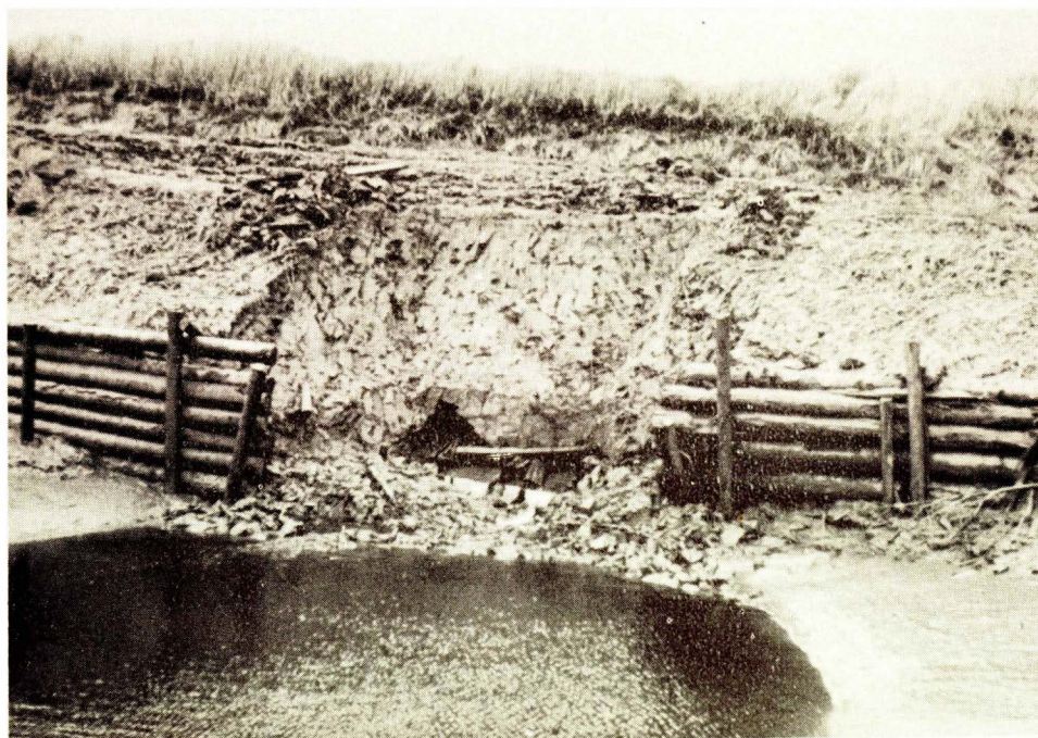
Fig. 6 - Project N. S. 5, Dugau Marsh, N. S. In order to determine the condition of this aboiteau outlet it was necessary to dig away the face. It will be noted that the down stream end of the sluice has collapsed, necessitating replacement of the aboiteau.
