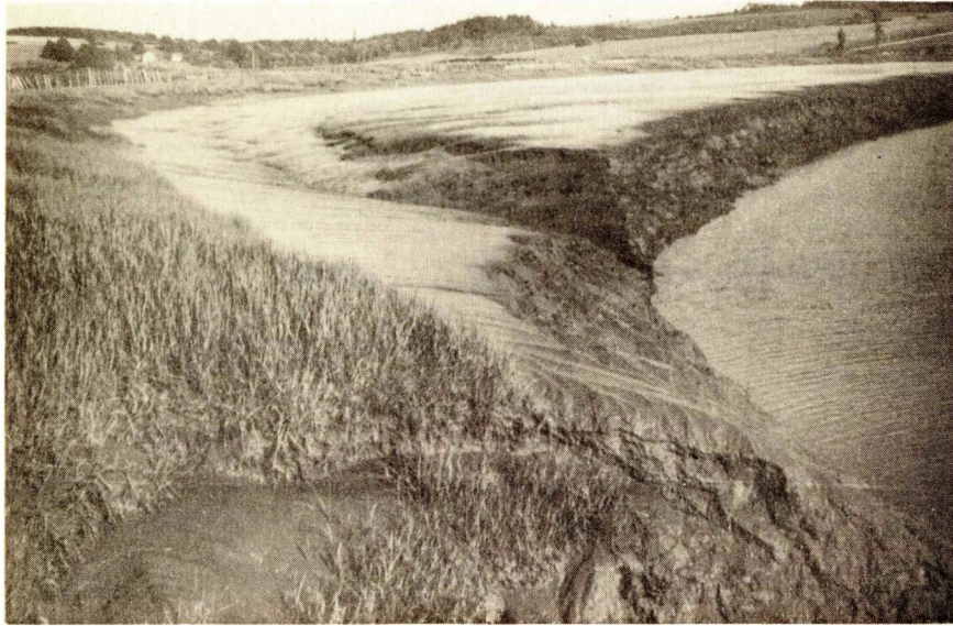
Fig. 23 - Project N. S. 49, Scotch Village Marsh, N. S. The dyke which is behind the poles on the right protects the Scotch Village Marsh. The tide water which flows up and down the Kennetcook River tended to undercut the bank on which the dyke was located. The erection of a small brush breakwater directed the currents away from the bank and the large silt deposit was thus encouraged.
