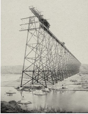
Lethbridge Viaduct under construction at tower 24. (United States Library of Congress's Prints and Photographs n.d.)
