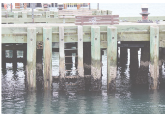
Barnacles mark the high water line on a pier
