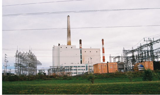
Trenton Generating Station - 307MW Opened in 1969
