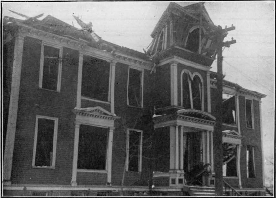
This is a view of the new Alexander McKay School. It now resembles a shell-torn building in Flanders.
