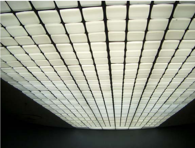
The lights in council chambers, very excessive lighting.
