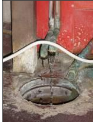
Figure 5. Outflow pipe of a typical cold room. Source: Paula Francis, 2007.
