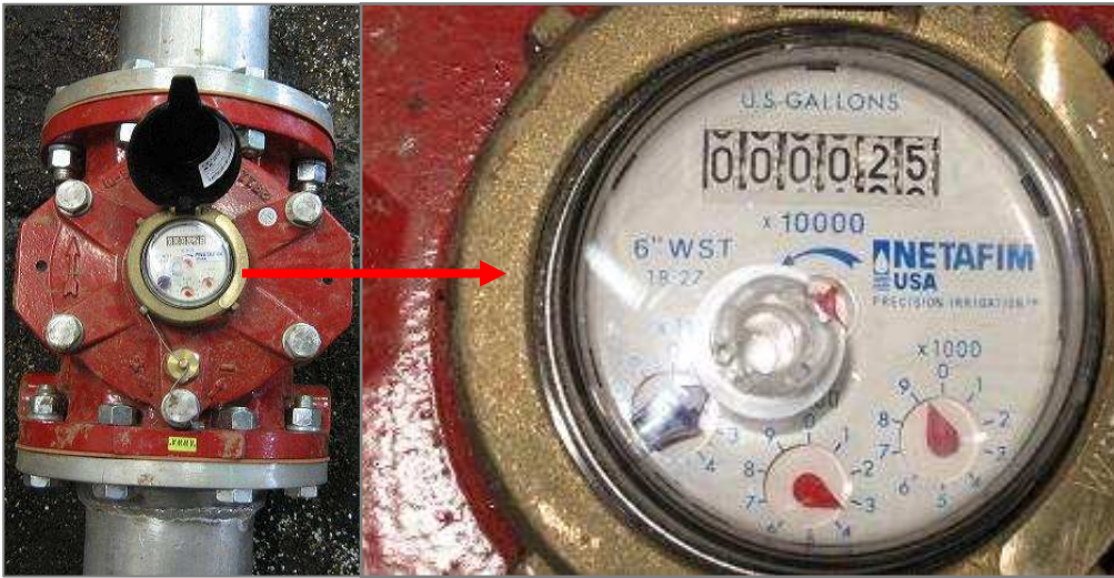
Figure 4.1: Water meter that is typically used to monitor water used for irrigation.
