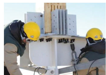
Bolted connections between structural members simplify on-site construction and reduce construction time; photograph by International Polar Foundation / René Robert
