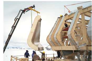
Panels are lifted into place at the Princess Elizabeth Antarctica Research Station; photograph by International Polar Foundation, “Passive Building Techniques”
