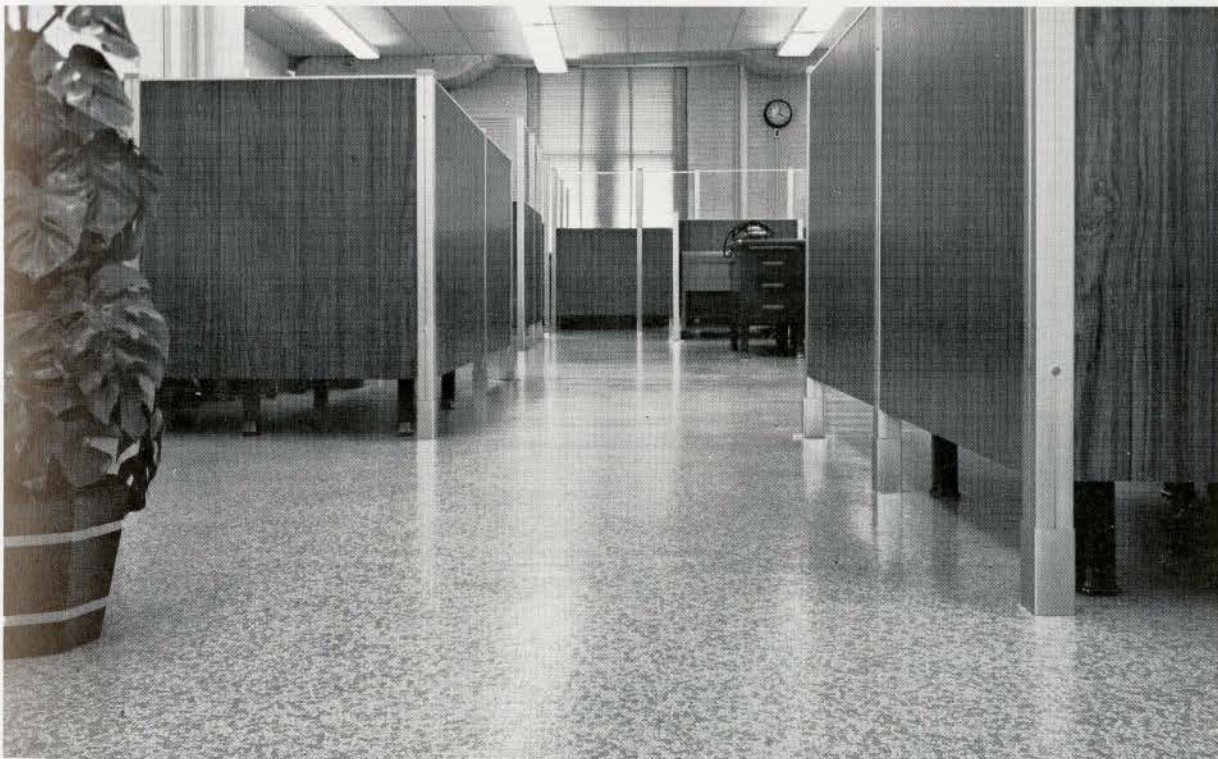
Below, new Tessera Corlon floor installed over old linoleum by time-saving Perimiflor System.
