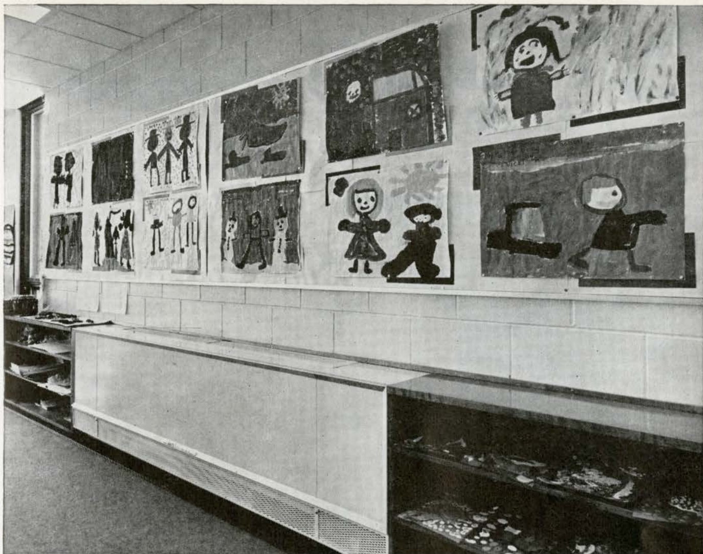
One of the electric unit ventilators at Redwood Public School. Architect: Jean-Paul St. Jacques, M.R.A.I.C. Consulting Engineer: Howard Boland, P.Eng.
