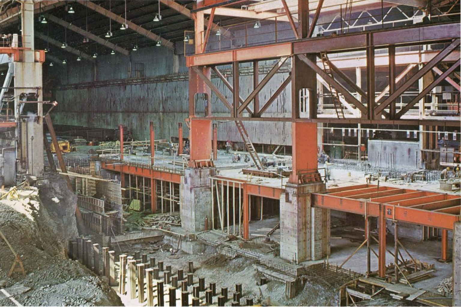
Piling for runout tables in foreground ; basement motor room in background. When completed, mill construction and equipment will be almost as extensive below ground as above.
