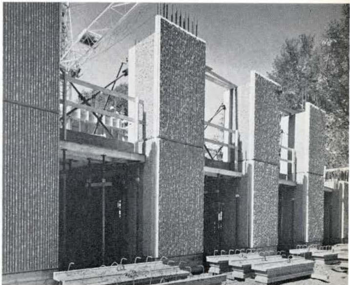
Panel is set on removable wooden shims, utilizing precision dowels for alignment and fast setting of panel above. After column is poured—shims are removed and open joint becomes expansion joint at every floor. No scaffolding required—building is finished on outside face after initial pour, eliminating need for formwork.
