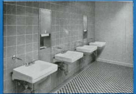
Typical Washroom Installation
