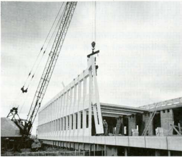
Research and Development Centre for the British American Oil Co. Ltd, Clarkson, Ont. Shore & Moffat and Partners, architects.
