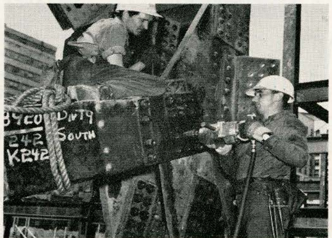
More than 1¼ million high strength steel bolts joined the components of Place Ville Marie's steel frame. This method ensured fast and quiet erection.
