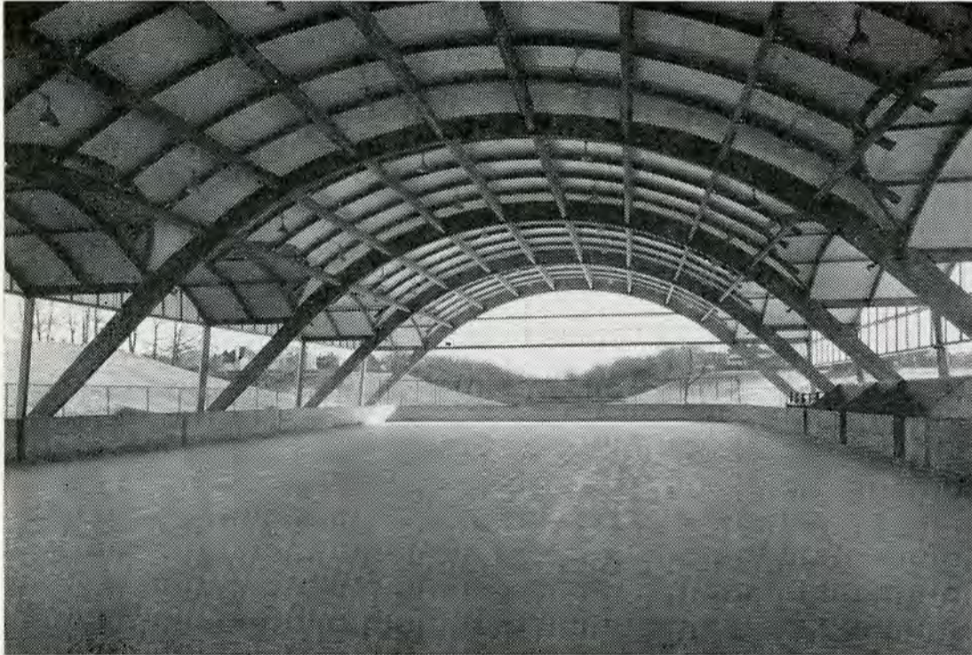
CEDARVALE ARENA — Contractor — Armien J. Martin Ltd., Toronto Consulting Engineer — R. E. Winter & Assoc., Toronto
