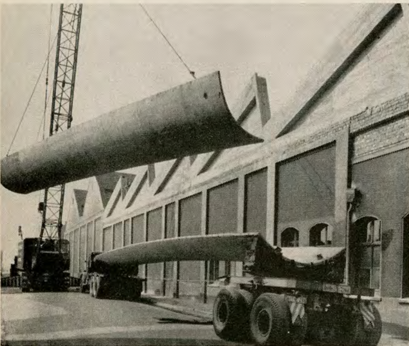
Top: hyperboloid, right, creates rotation surface for 54-ft-span roof shells, covering 12,750 sq ft, at Pertrix Battery Plant, Frankfurt. Center: mold ready to receive. Bottom: erecting roof shell.
