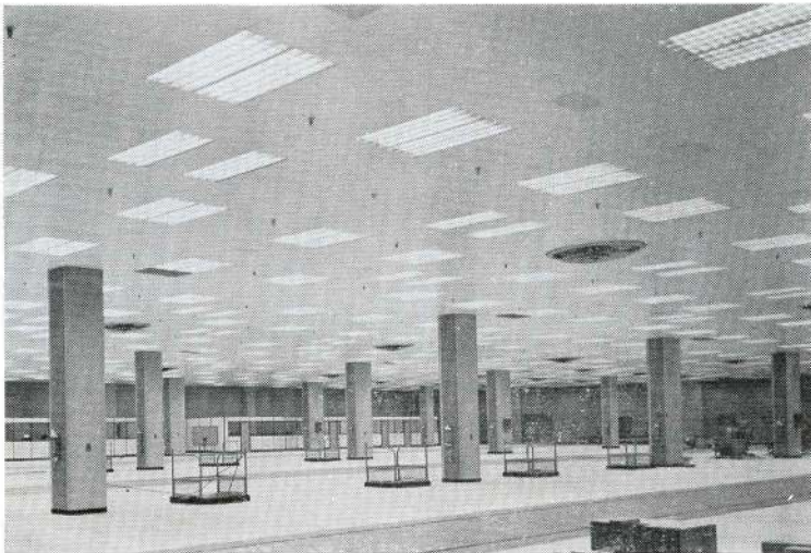
Imperial Tobacco Company of Canada, Limited, Guelph, Ont. Installation 4 lamp 2' x 4' LBQ Troffers Average Illumination Level — 75 Footcandles Architect: McDonald & Lenz, Hamilton Consulting Engineer: R. R. Allsop & Assoc., Toronto Electrical Contractor: Canada Electric Co. Ltd., Toronto
