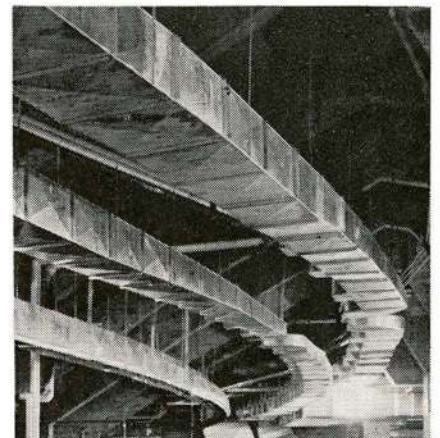
Galvanized Duct Work
