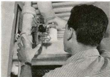
This Edwards Waterflow Switch activates the fire alarm system when any of the buildings' sprinklers go into action.
