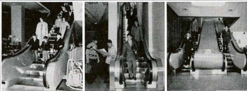
One of many store installations across Canada, Turnbull Escalators provide safe uninterrupted service between department floors in the Simpson-Sears Winnipeg store.
