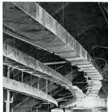
Galvanized Duct Work
