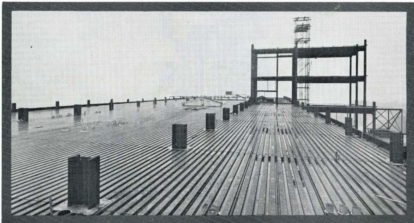
Q-Roof deck of Lion's Gate Hospital, Vancouver, B.C. Architects: Underwood, McKinley & Cameron
