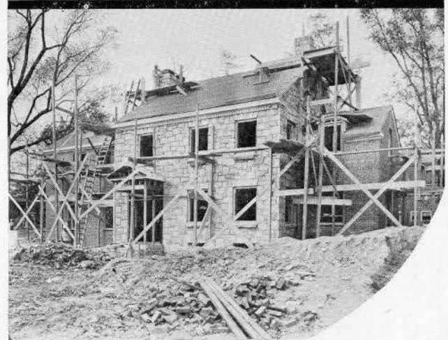
Note brick and stone facing applied over TEN/TEST sheathing.
