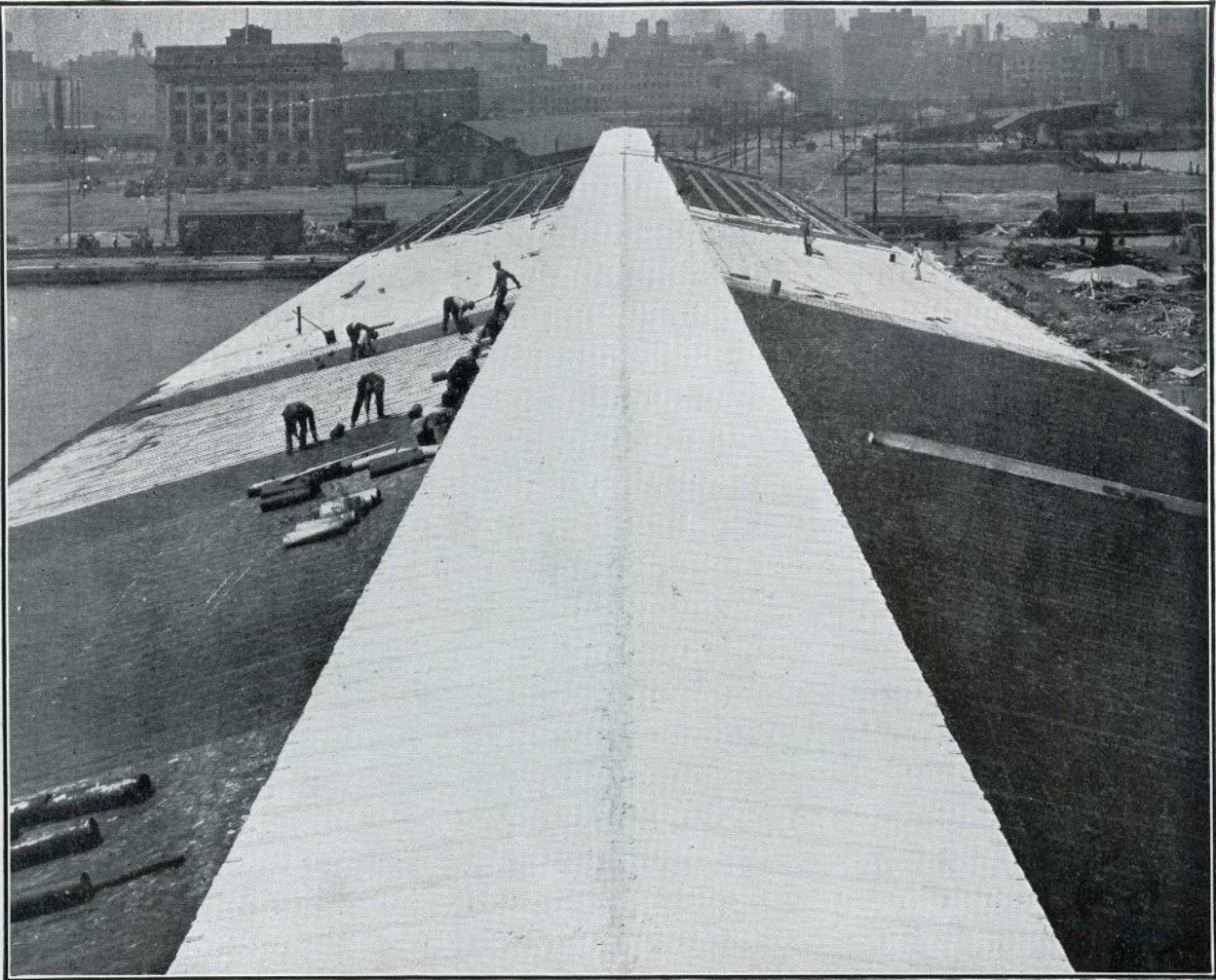
Roof of Canada Steamship Freight Sheds, showing Long Span pre-cast gypsum roof slabs being applied. Carswell Construction Co., Ltd., Engineers. Jackson and Lewis Co., Ltd., Contractors.
