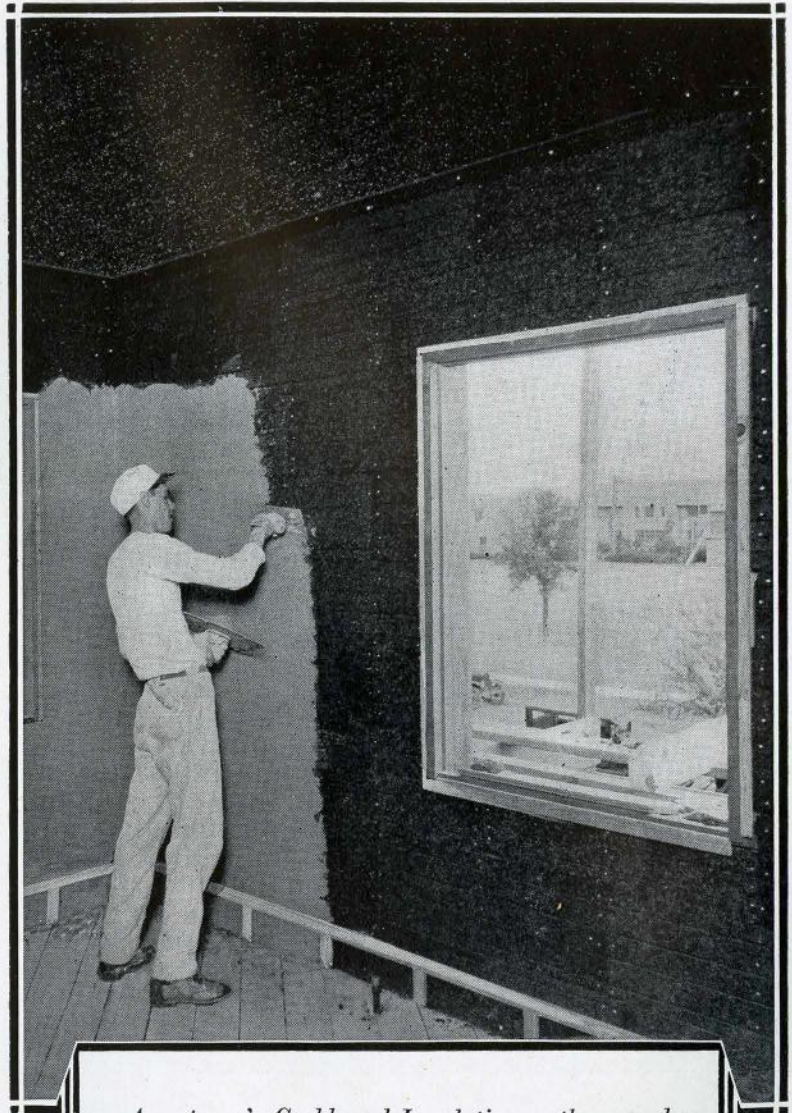
Armstrong's Corkboard Insulation on the second floor of Mr. H. B. Thompson's residence at Dallas, Texas. The plaster is being applied directly on the cork, without lath.
