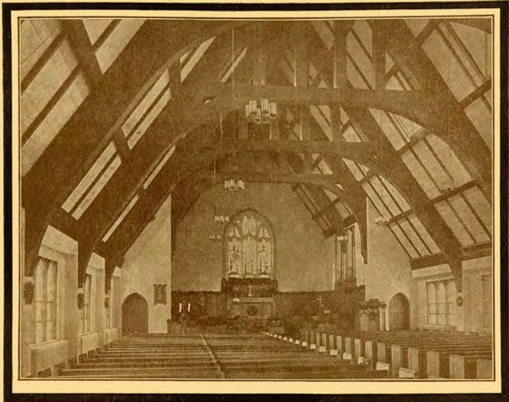
Armstrong's Corkboard installed between the rafters of St. Mark's and St. John's Episcopal Church, Rochester, N. Y.
