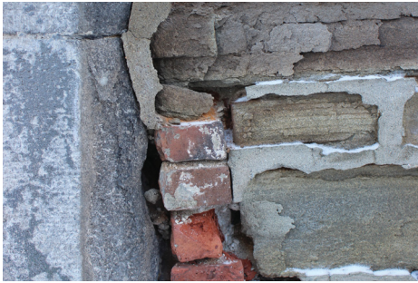
Damage to the façade of Caserne 7
