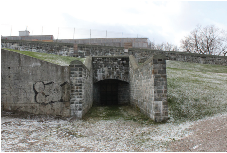
Poternes along the fortification wall are reopened to provide connection points between the Institut Nazareth and the Hôtel-Dieu.
