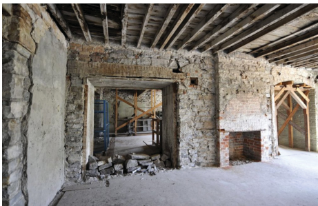
Damage to the interiors of the Nouvelles-Casernes (from Steve Deschênes, 2012)
