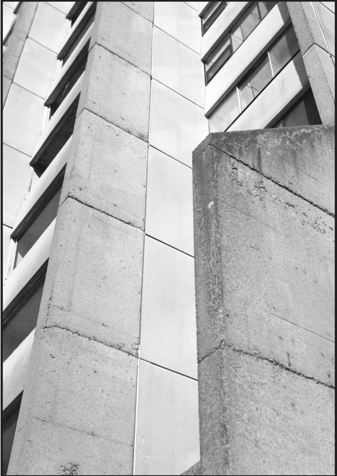
Fig. 52. Photograph of the structural fins of Fenwick Place. The associations to the Unité d'habitation are legible in the materiality of the unfaced concrete and the heroic scale and expression of the structural forms.
