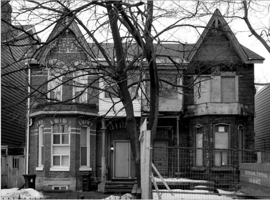
FIG. 29. HOUSE ON BERKELEY UNDERGOING FAÇADE RECONSTRUCTION, SHOWING THE WOOD PLANK BACKING OF THE DECORATIVE SINGLE WYTHE BRICK VENEER. THIS FAÇADE'S BRICKWORK HAS BEEN REBUILT TO MATCH THE ADJACENT HOUSE. | SCOTT WEIR, 2015.
