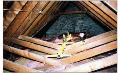
FIG. 26. ST. JOHN'S, PORTSMOUTH, ROOF AND SCISSOR BEAMS BETWEEN THE PLASTER CEILING AND THE ROOF TOWARD THE EAST. | FRED CRAVEN, 2011.
