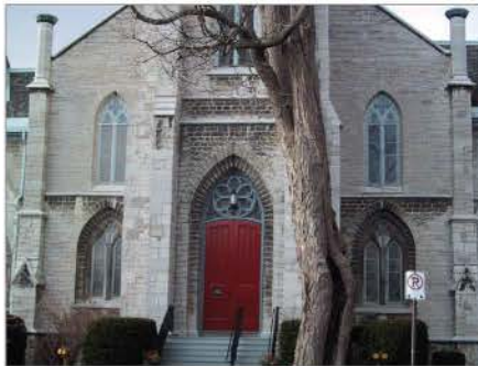
FIG. 30. SYDENHAM STREET UNITED CHURCH (1852), KINGSTON, STONEWORK OF THE ENTRANCE FAÇADE. | PAUL CHRISTIANSON, 2006.
