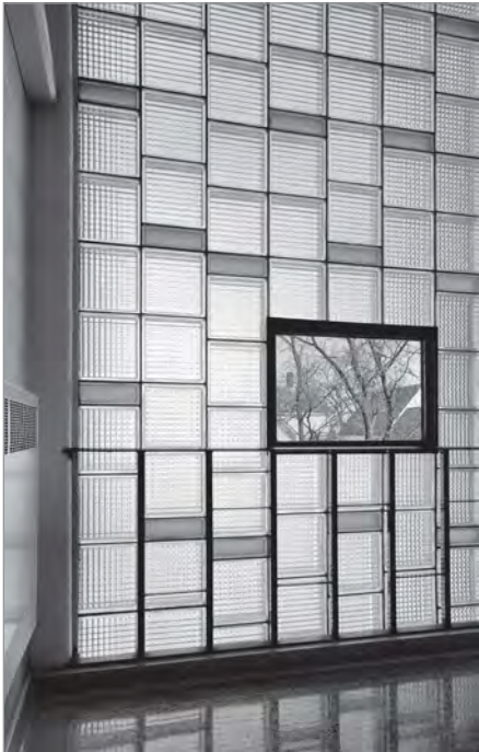
FIG. 6. CLASSROOM ANNEX STAIRWELL GLASS BLOCK WINDOWS, FORMER FREDERICTON HIGH SCHOOL, WILLIAM LAKE, ARCHITECT, 1961. | JOHN LEROUX.
