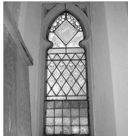
FIG. 19. ST. JAMES' DETAIL OF WINDOW FROM THE SIDE ENTRANCE PORCH. | PAUL CHRISTIANSON, 2014.
