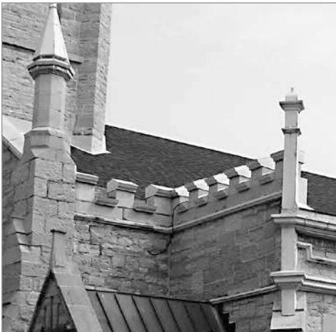
FIG. 22. ST. JAMES' DETAIL OF PINNACLES AND BATTLEMENTS ON ADDITIONS OF 1888-1889. | PAUL CHRISTIANSON, 2013.
