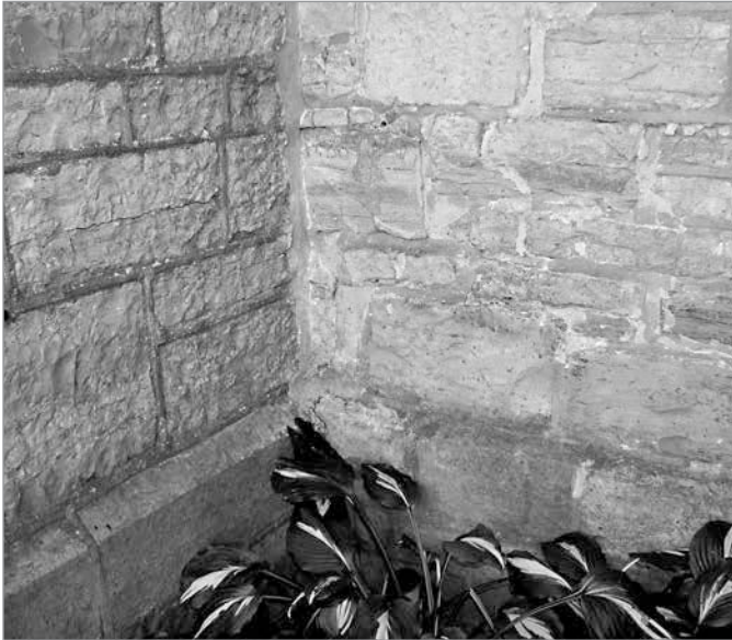
FIG. 14. ST. JAMES' DETAIL OF THE NEW AND ORIGINAL PLINTH COURSES AND STONEWORK. | PAUL CHRISTIANSON, 2013.
