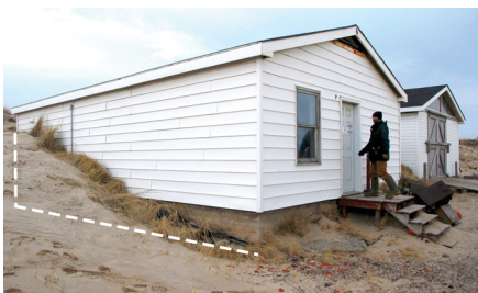
This is accelerated when the structure is in the path of an advancing dune system. The generator and storage facility at West Light is being rapidly consumed by the advancing north dune.
