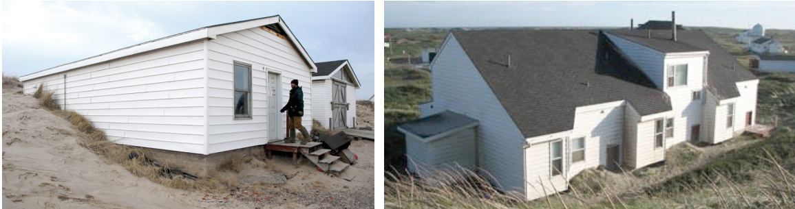
Images of sand engulfing buildings at west light (left) and Main Station (right), Sable Island, 2011, photographs from Parks Canada
