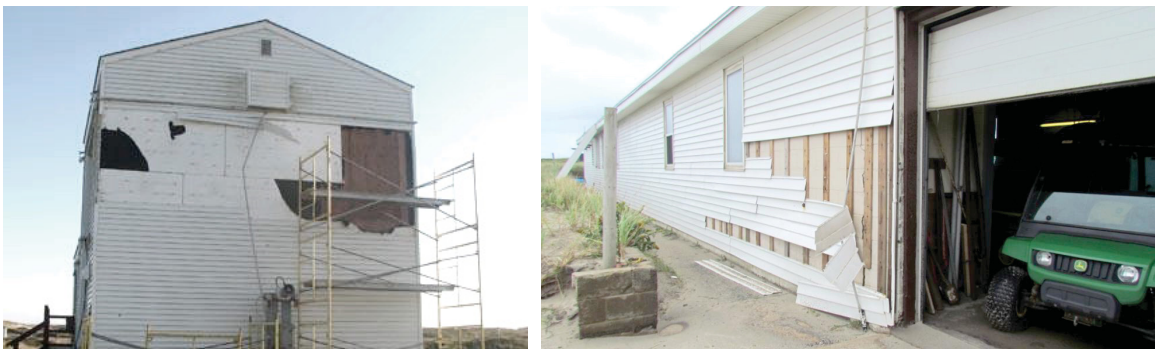
Images of vinyl siding being blown off of buildings at Main Station, Sable Island, 2011, photographs from Parks Canada
