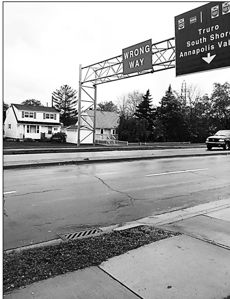
Figure 2-12 Consistently spaced thermal transverse cracking, photo taken at Bayers Rd. toward Highway 102 North, Halifax, Nova Scotia, October 27 th 2013
