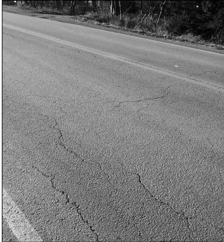
Figure 2-10 Early stages of fatigue cracking formation, photo taken at Old Sambro Rd, Halifax NS, October 29, 2013
